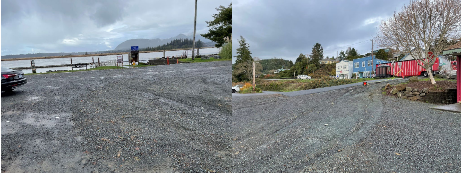
Driveway to gravel paved lot at Waterfront Park. This area is used for people to walk between the town, park and dock. Recent heavy rains caused flooding and damage to the driveway and pathway into the park.
