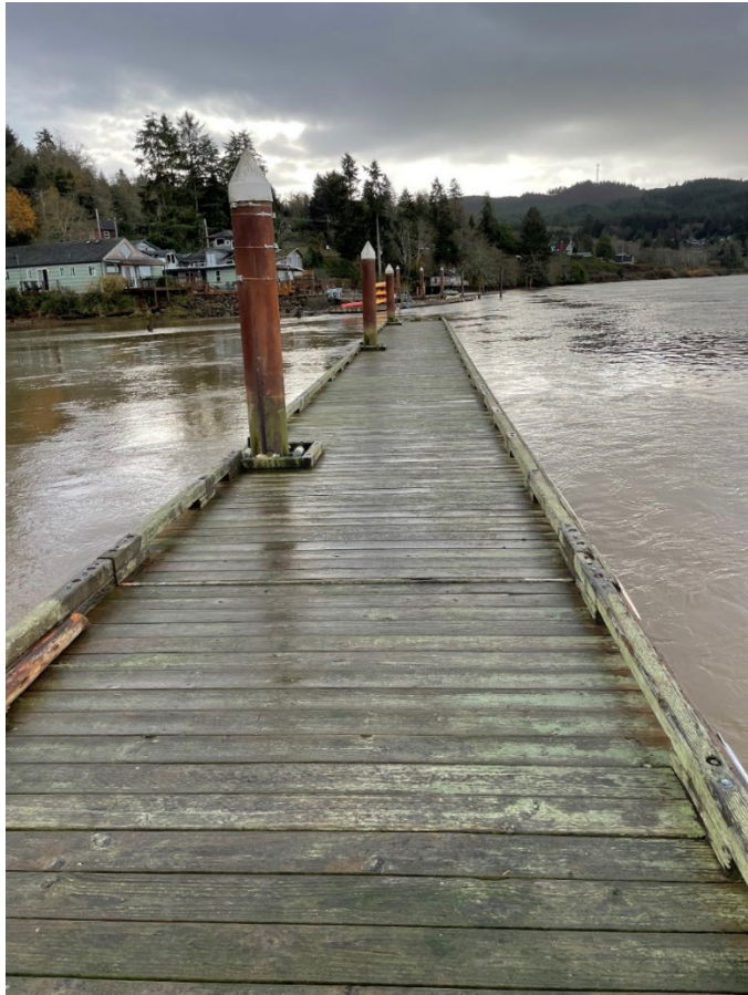
Dock- wet, slippery wood.
