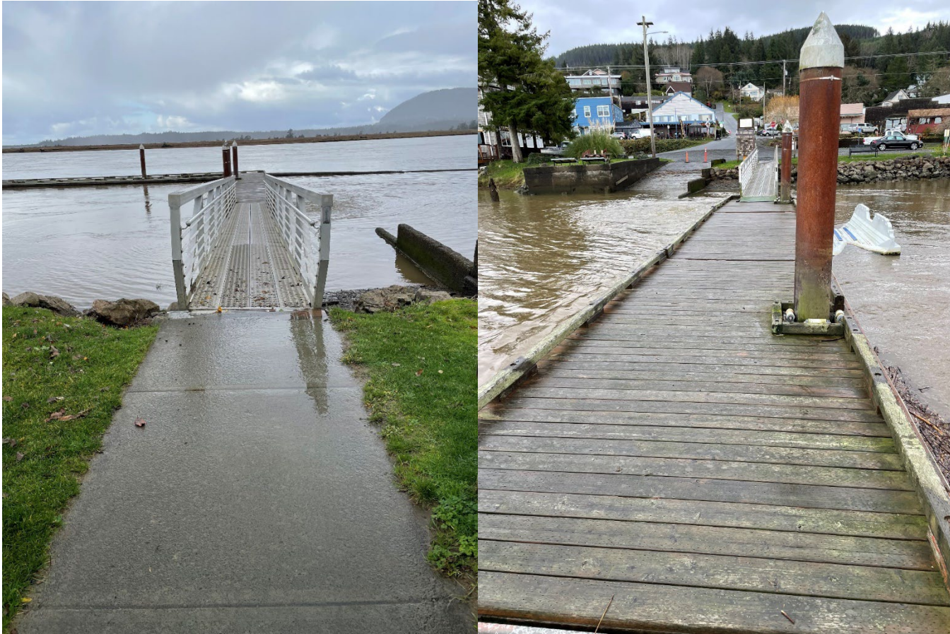
Gangway to dock, kayak lifter on the side of the dock. The gangway is metal grating and leads to a wood dock. The wood is wet, slippery and showing signs of wear.
